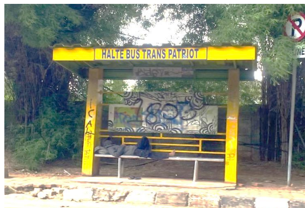
Figure 2. Condition of Trans Patriot Bus Stop, Bekasi City
