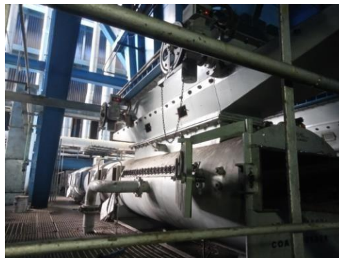
Gambar 1. Coal Feeder PLN UPK Nagan Raya
